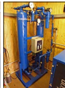
Air Dryer (for sparging air)
