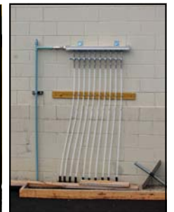
Sparge Well Manifold (remote from system)
