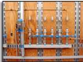
Air/Ozone Flow Control Valve and 6-well Sparging Manifold
