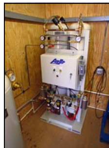
Oxygen Generator (ozone generator feed gas)
